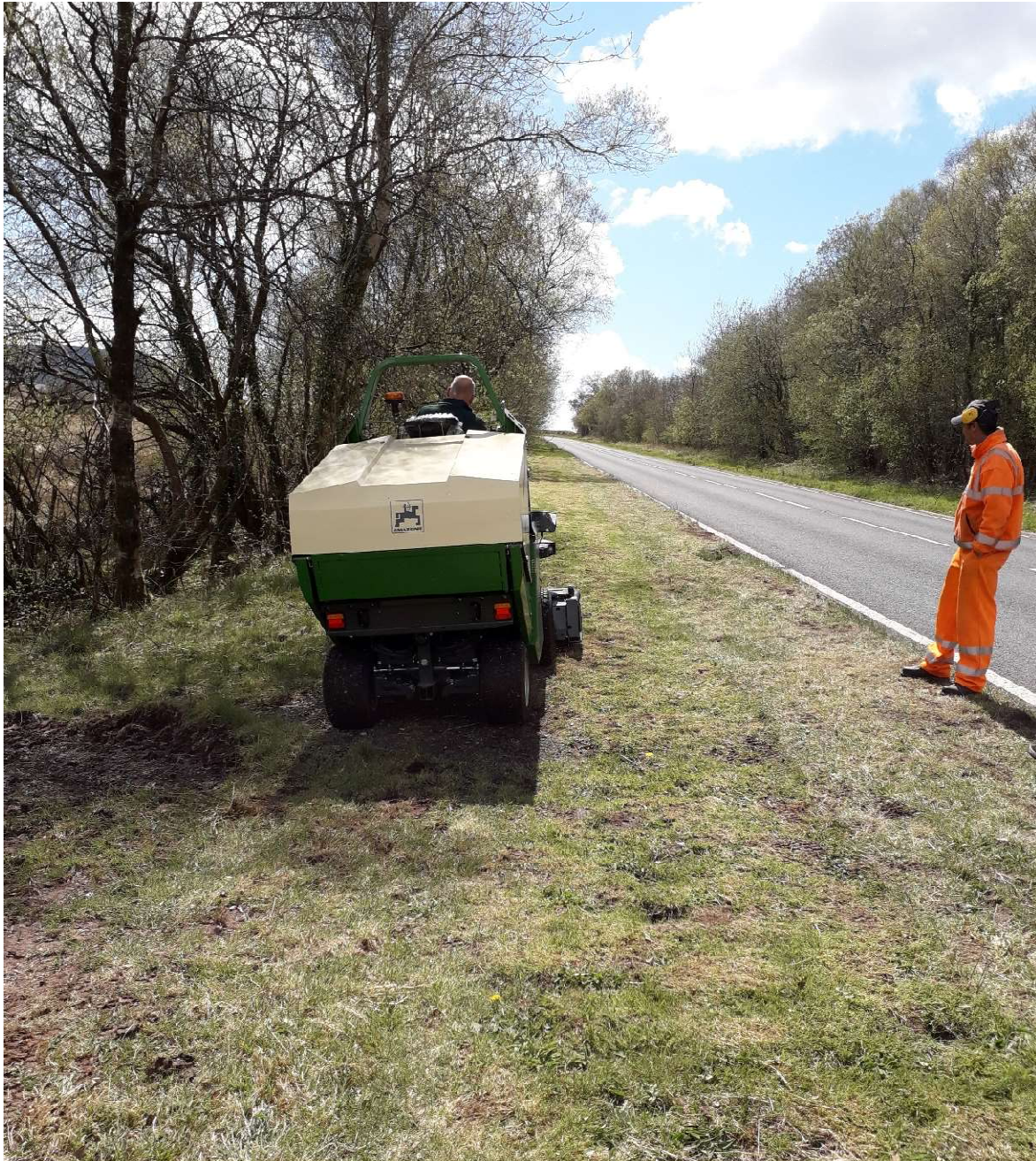
FIGURE 2.1: CUT & COLLECT MACHINE USED BY HIGHWAYS TO MANAGE ROADSIDE VERGE NATURE RESERVES (RVNRs).
